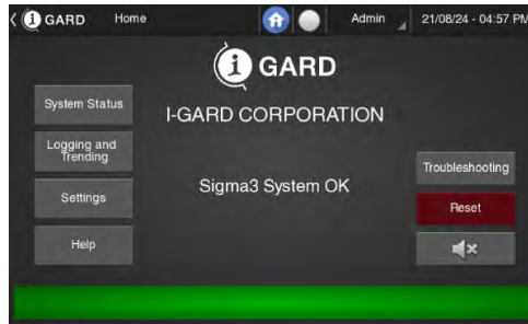
Figure 5: Sleuth Control Panel / TDM Home Screen
