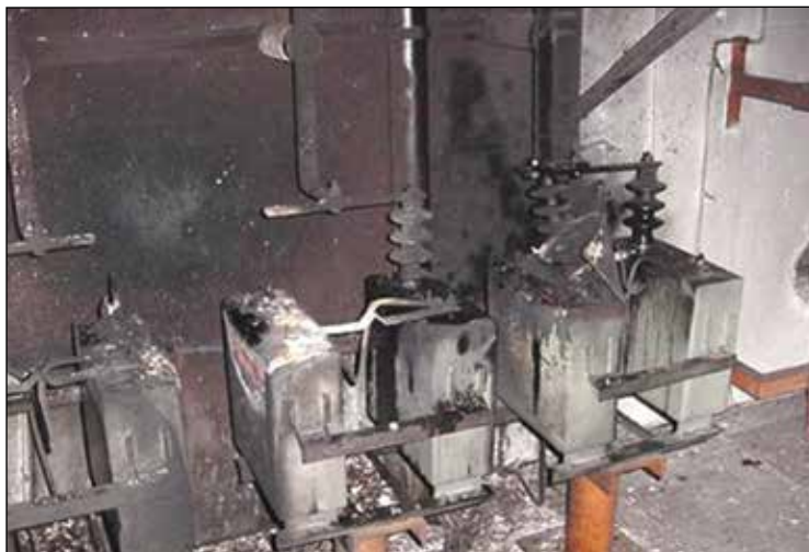
Figure 1. Ungrounded system burn-down damage
