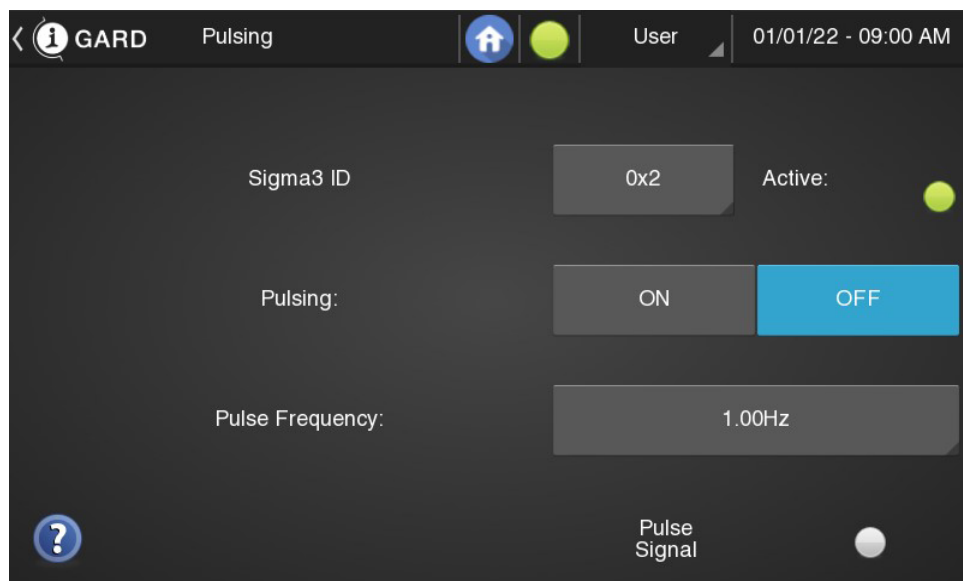
Figure 7.7: Pulse Contactor Settings Screen
